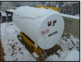
Skidded Westeel fuel tank
